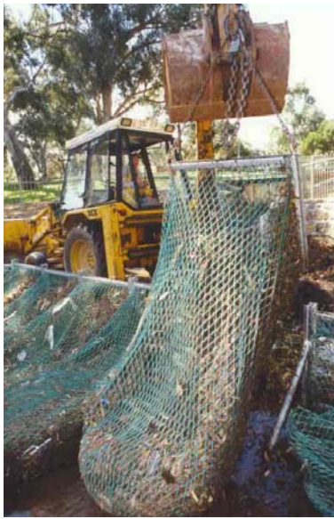
Figure 9.10 Clean Out of GPT Baskets Across Third Creek, Adelaide
