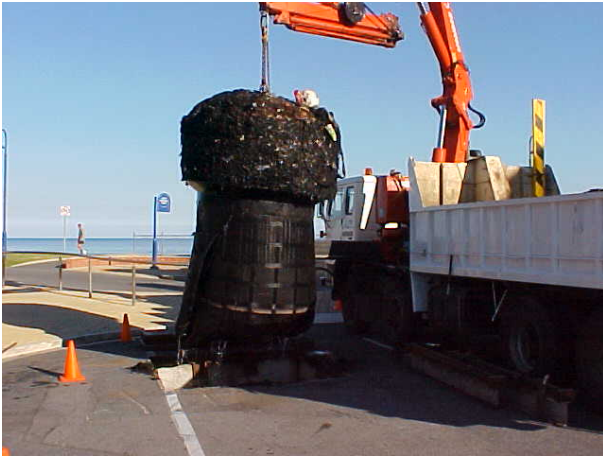
Figure 9.16 GPT Maintenance - Pier Street, Glenelg
