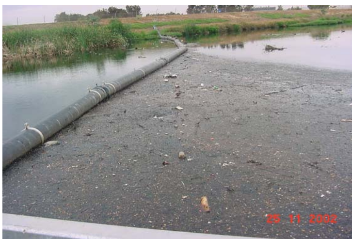
Figure 9.11 Floating Boom Operating at Netley, West Adelaide
