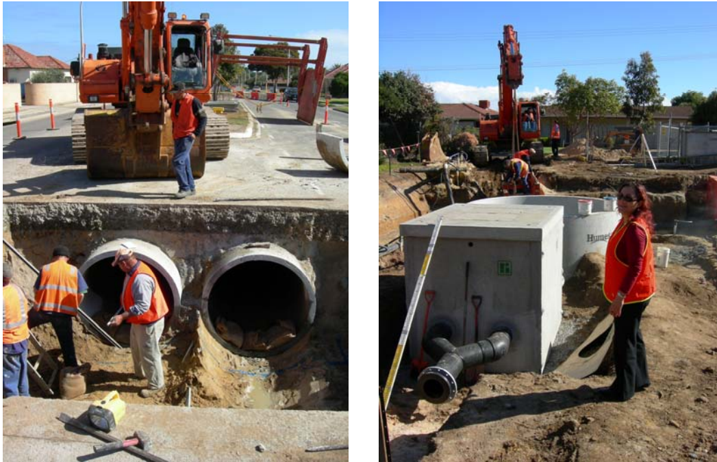
Figure 8.5 Grange Golf Club Stormwater Harvesting and Reuse Scheme - Trimmer Parade Diversion and Frederick Road Pit (August 2006)
