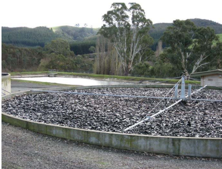
Figure 14.1 Gumeracha Wastewater Treatment Plant
