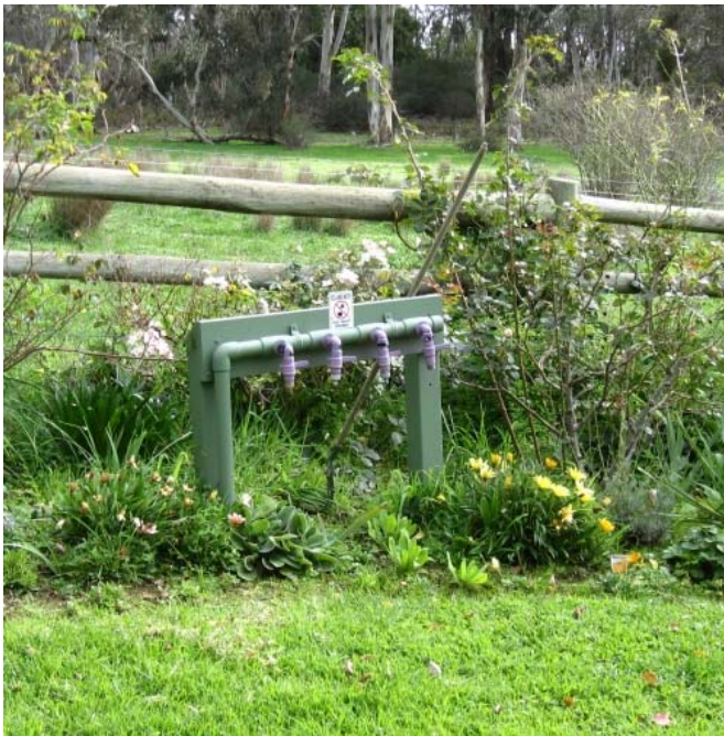
Figure 14.2 Treated Wastewater from the Hahndorf WWTP Utilised at The Cedars
