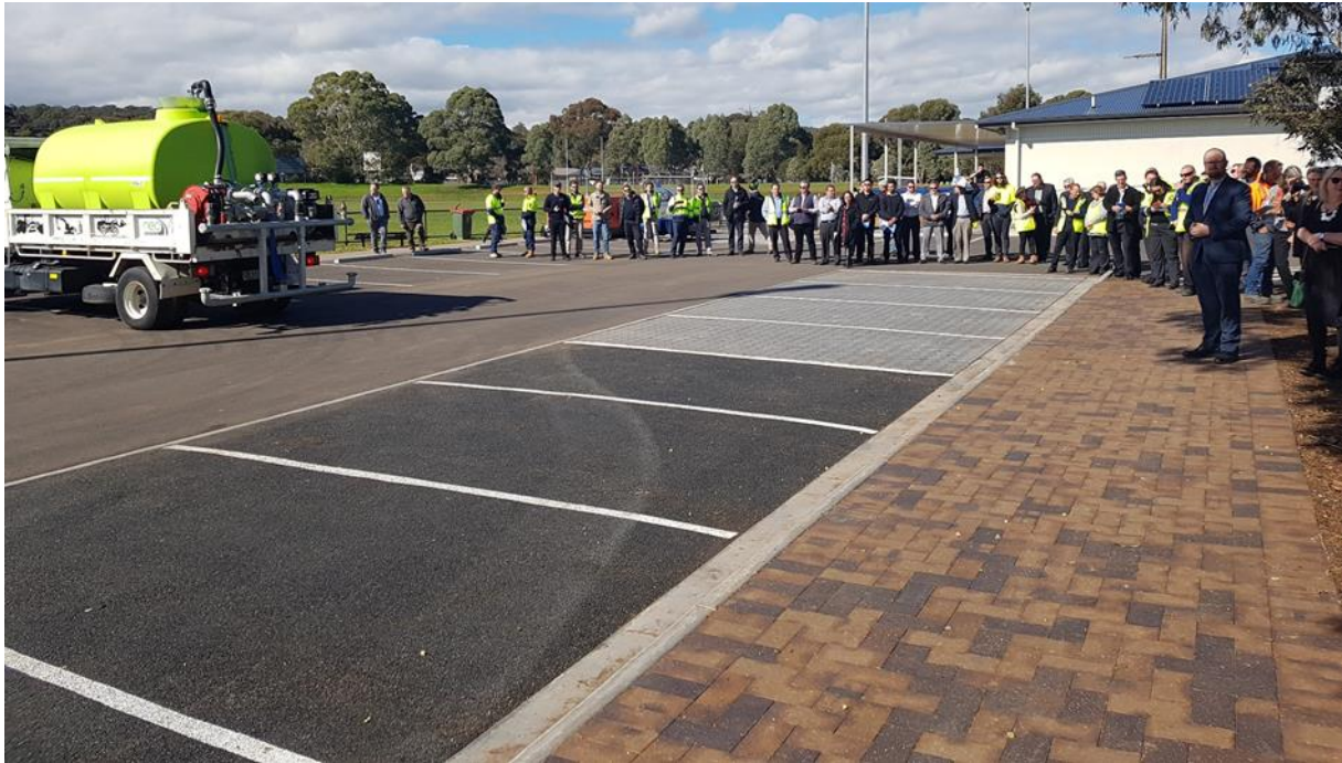
Figure 6.13 City of Mitcham, St Marys Park carpark, crumb rubber porous asphalt and permeable paving trial
