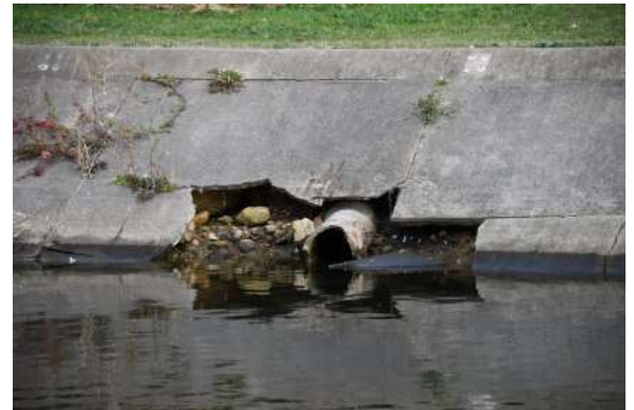
Failure of concrete batters
